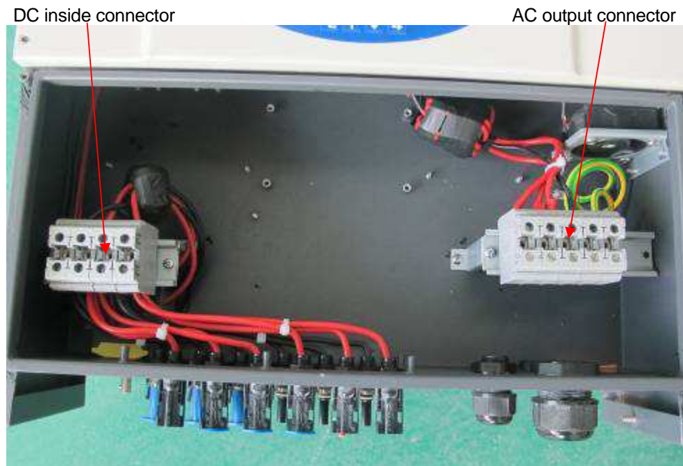
Internal view of the unit
